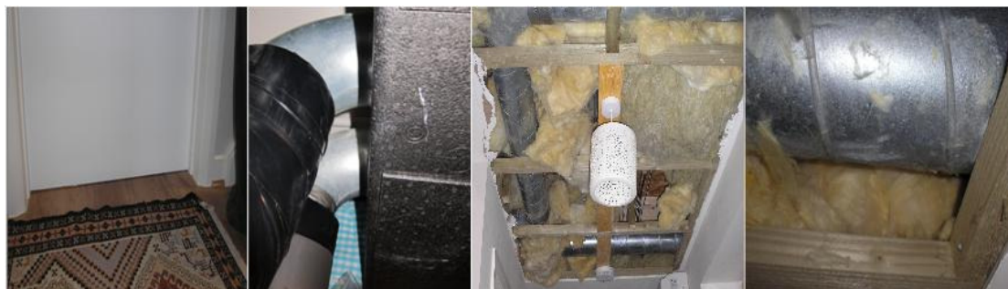
Figure 3. Issue with the ventilation system: missing transfer openings under doors, missing and inadequate cold duct insulation, moisture problems due to inadequate insulation and sealing of cold ducts required ceilings to be opened.
