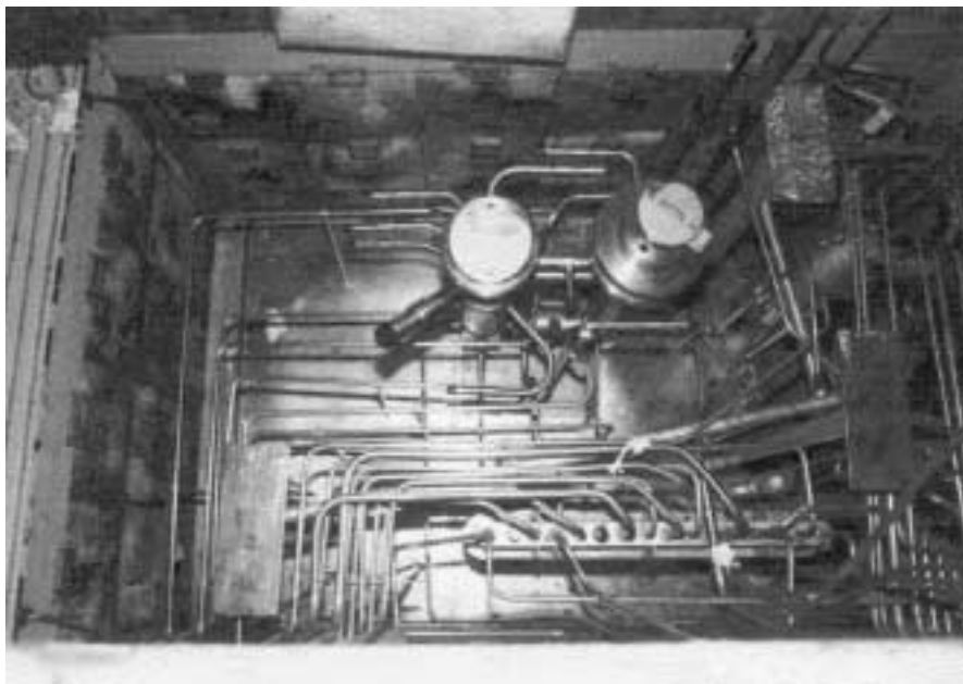
Figure 11. Photograph showing titanium dissolver assembly with piping.
