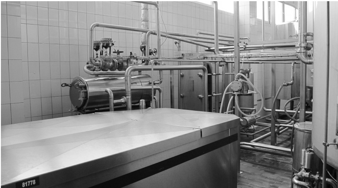
Fig. 1. General view of the pasteurization machine № 2
