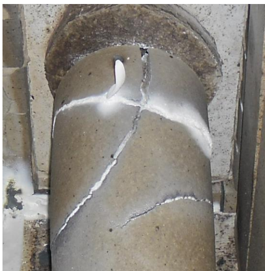
Fig. 1. Cracks on the connecting channel in the manufacture of zinc oxide. (full colour version available online)
