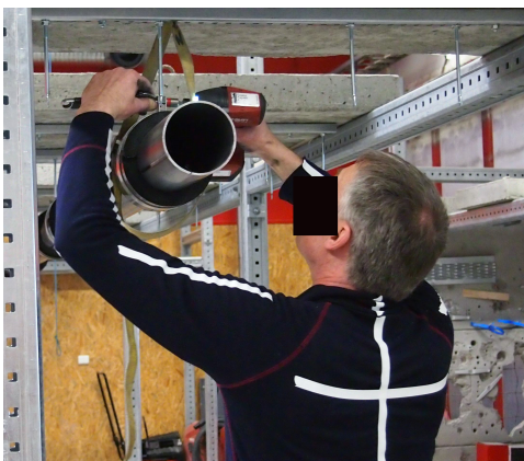
Figure 6.11 Screws on top of the pipe, system 1
