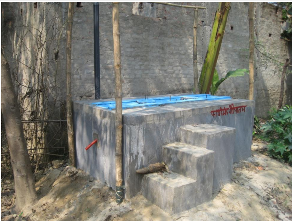
Photo C – A UDDT under construction. The substructure has been built while the frame for the superstructure has been started.
