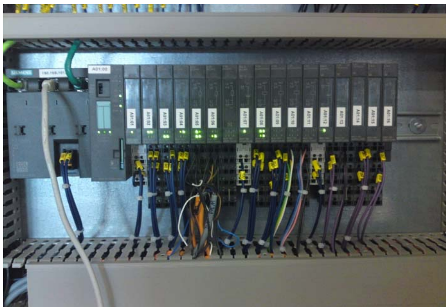
Figure 9: PLC and I/O modules.
