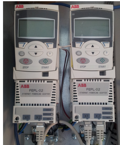
Figure 2.7: The VFD's with mounted external modules
