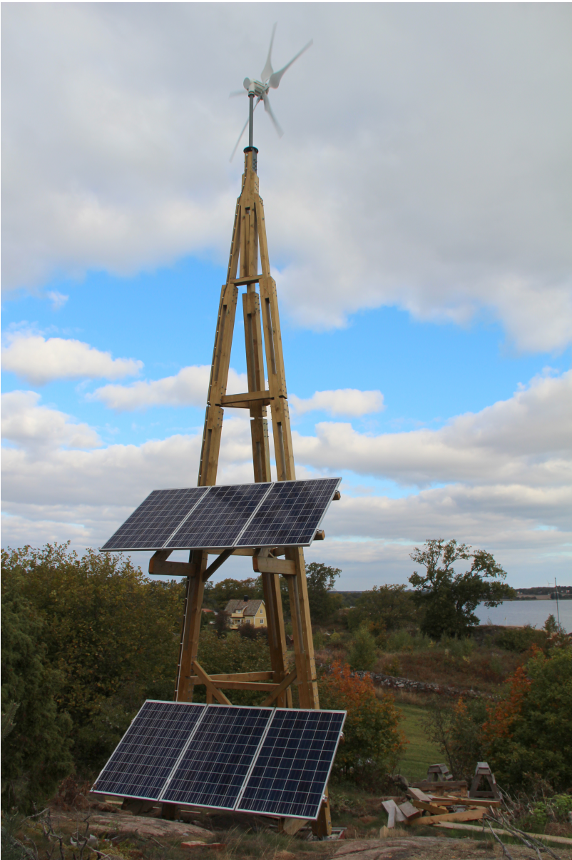
Picture 1. The Dali PowerTower (source: InnoVentum AB, 2013b)
