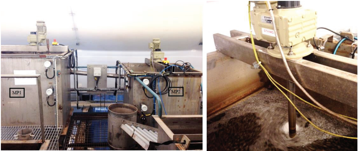
Figure 3-3. Reactors MP1 and MP2 (left) and MP2 (right) in the Manamnox pilot plant.
