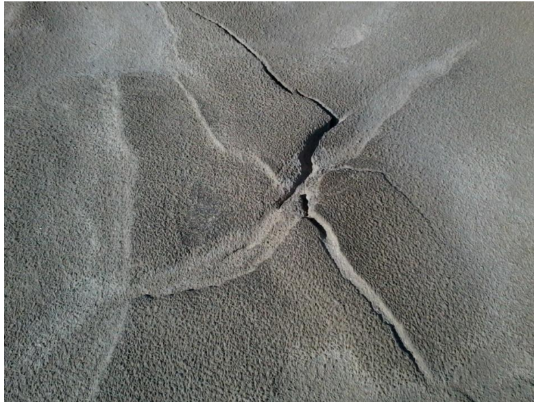
Figure 5-7: Dry crack in surface of the tailings dam approximately 250 m out in dam A 2013-09.
