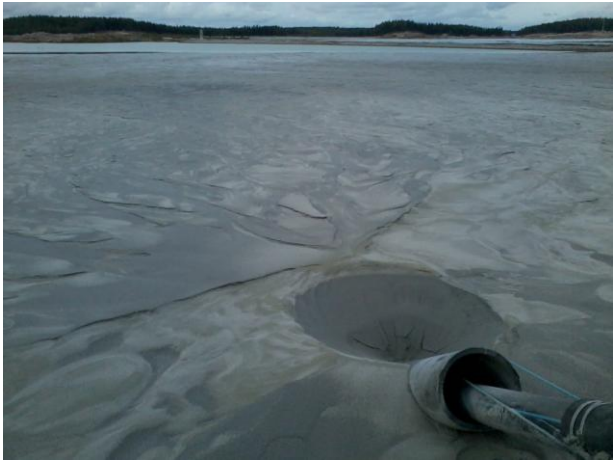
Figure 5-20: Beach at dam C section 1+850, 2013-09.
