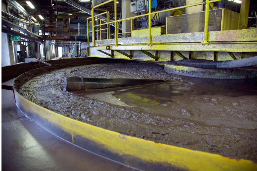
Figure 2-2: Sedimentation basin in the extraction plant at Garpenberg (H. Aitahmed-Ali (Boliden), personal communication, 2013-10-31).
