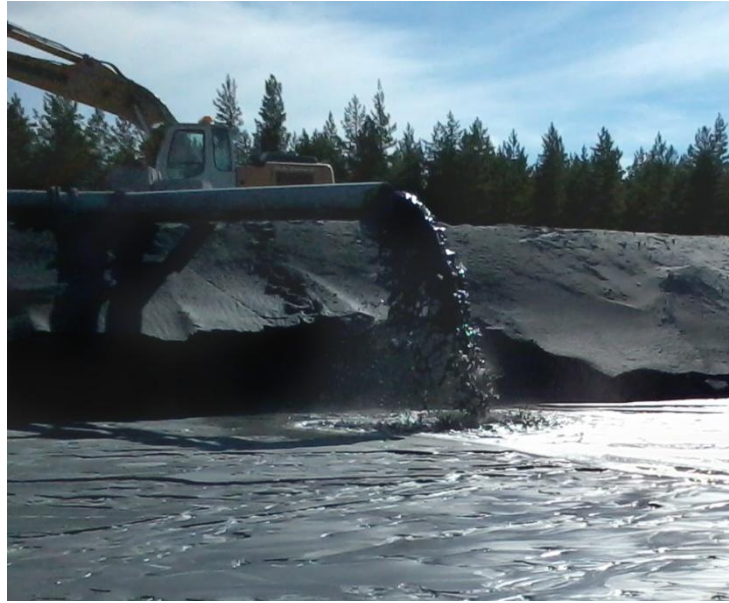
Figure 2-5: An open end pipe at the Garpenberg tailings dam 2013-09-03.
