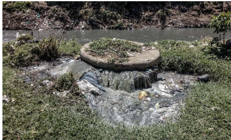
Figure 11: Broken Sewer Line in Slum Area . Nobody expects the government to fix things like this, which expose slum dwellers to 'imported' risks from other areas.
