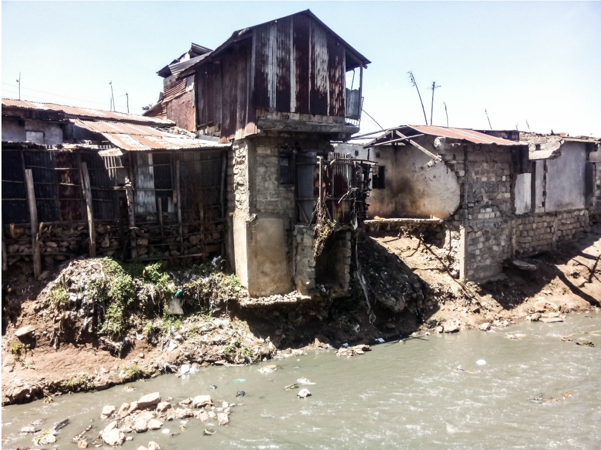
Figure 9: Riparians in Slum area are most affected by annual floods. Recent high-waters have flushed away parts of this building in Dandora. Source: Own.
