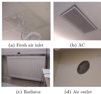
Figure 2.4 HVAC components in the test-bed. [KTH-HVAC-Wiki, 2015]
