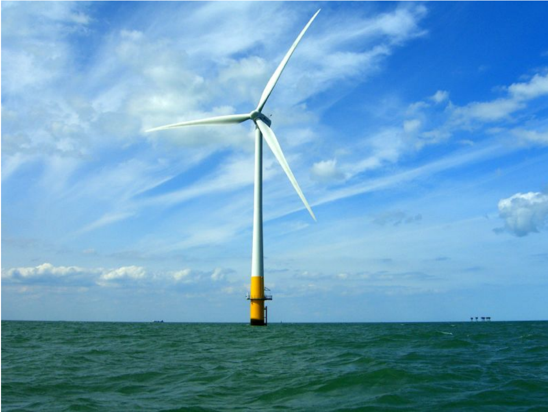
Figure 3.3: Vestas V90 turbine
