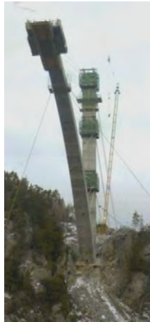
Figure 13 - Cantilevering method applied in the construction of the arch rib using an auxiliary pylon
