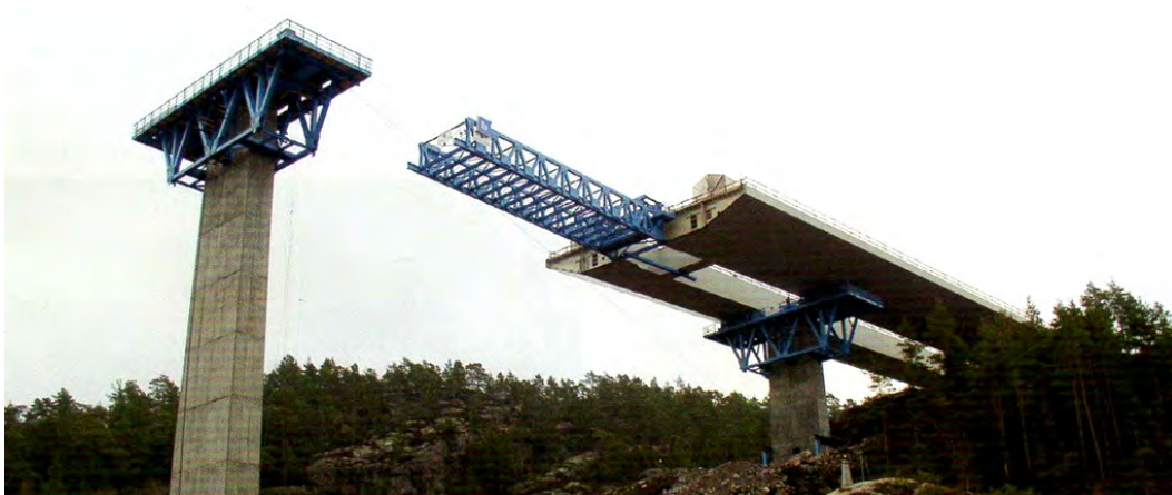
Figure 16 - Incremental launching using the movable launching nose - Construction of the superstructure from the Swedish side
