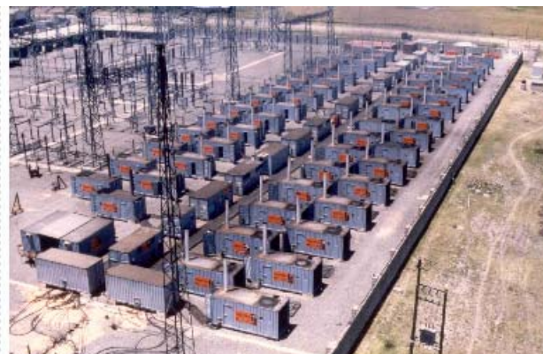
Figure 21: Aggreko Diesel Plant
