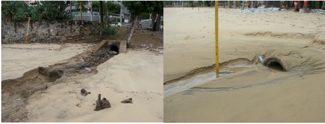
Figure 14. Storm water outlet pipes located on the adjacent beach. (Photos: Seth von Dardel, 2015)
