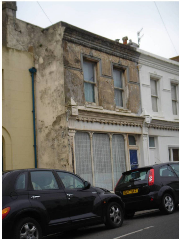
Plate 5.5: Photo showing run-down property on Norman Road
