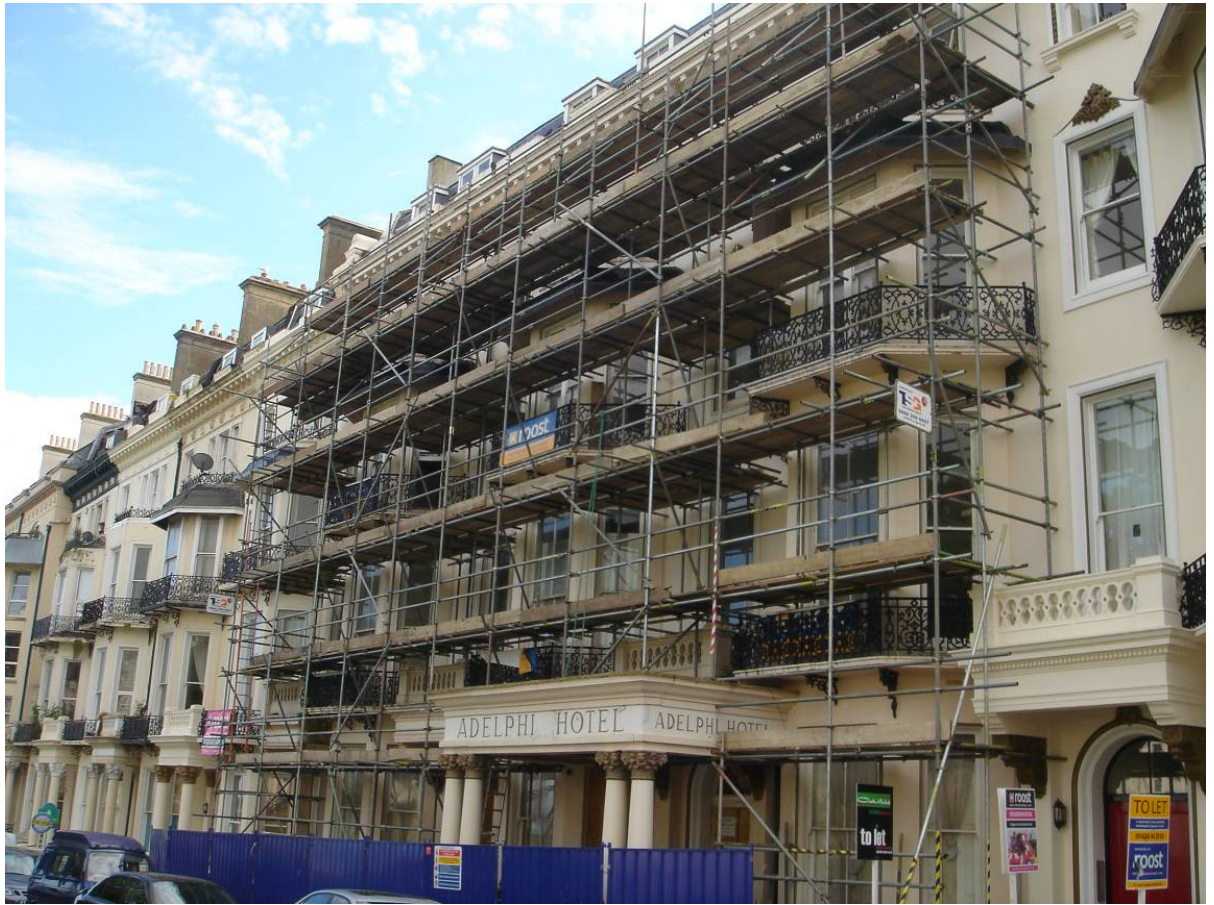
Plate 5.4: Renovation works on the Adelphi Hotel in 2008 (prior to it being used as student accommodation).
