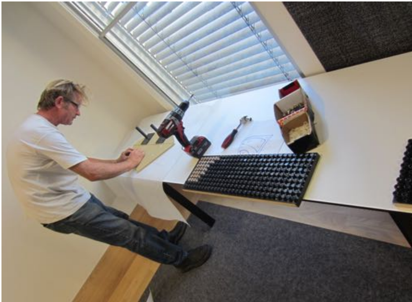
Figure 2.54 Brackets fixed to back of painted panels in preparation for wall installation Photo – ©Simon Perry
