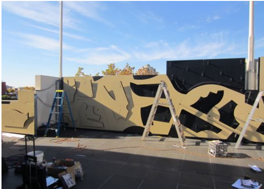
Figure 2.55 Artwork panels installed and fixed onto steel wall by Derek John of D.J Projects Photo – ©Simon Perry
