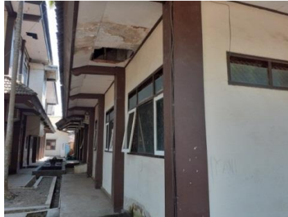
Figure 1: Condition of structural elements of the IAIN Jember employment building
