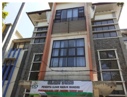
Figure 4: The condition of the structural elements of the post-graduate building in IAIN Jember
