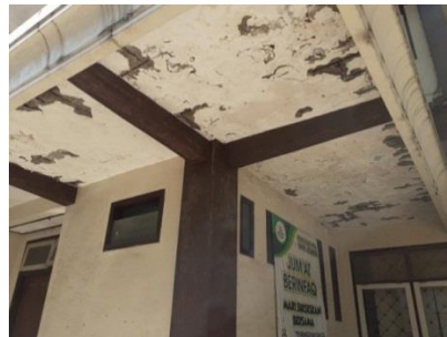
Figure 2: Condition of structural elements of the IAIN Jember lecture building
