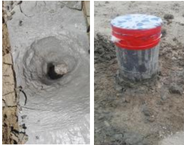
Figure 6. Construction steps of single jet grout soil-cement column (D=150 mm and L=2000 mm)
