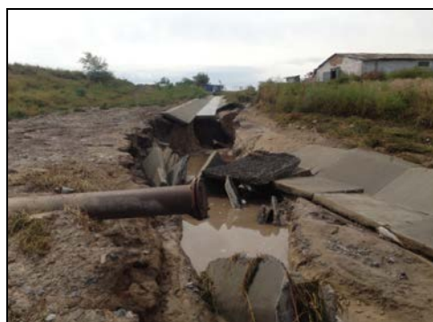
Fig. 5. Displaced concrete ditch downstream the red sludge pond
