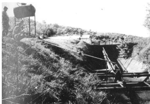
Figure 9 The pumping microstation Mocrea, Ineu, Arad county, Romania
