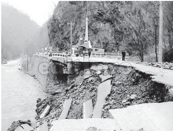
Figure 6. Bank's collapse and asphalt's damage (www.editie.ro), near the confluence Polatiștea-Jiu, at km 121+ 272
