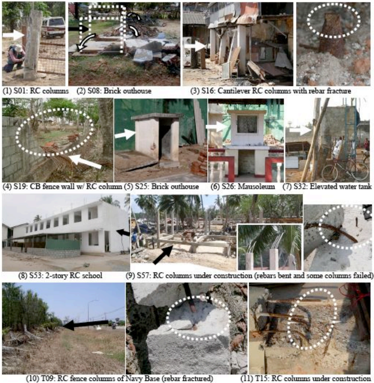
Photo 1 Typical damage to investigated structures ("S01" etc: ID Nos. in Table 1, "→": tsunami flow direction)
