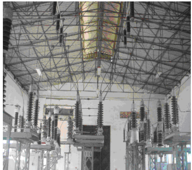
Figure 1. View of the 66kV enclosed air substation at Linoperamata
