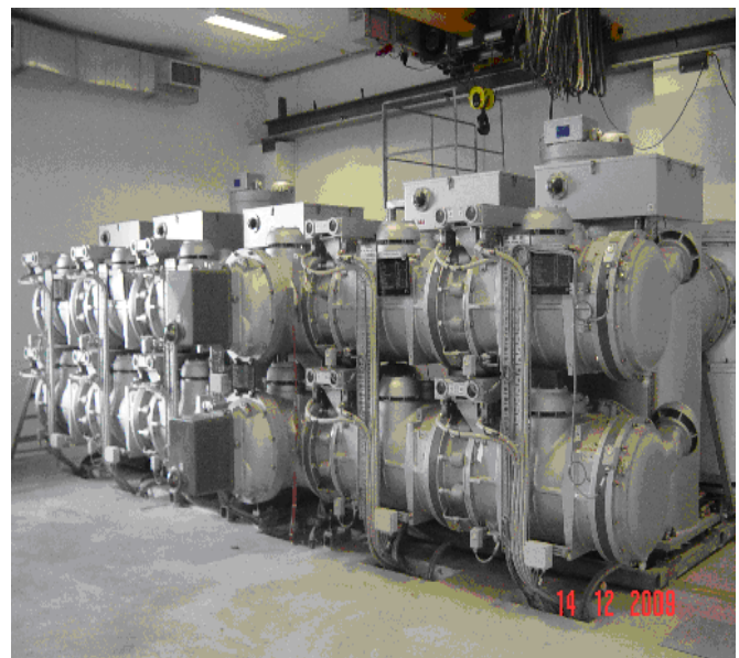
Figure 2. View of the 150kV GIS at Heraklion Crete
