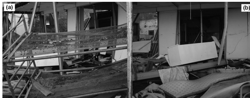
Fig. 12. Two pictures of building #5 (Punta Lena, Stromboli – Fig. 6) taken after the 2002 tsunami. The flow broke doors and windows, penetrated indoors and dragged the building contents outside (a). A large crack can be observed in the front side wall (b). However, that wall does not appear to be part of the load-bearing structure of the building, as does the undamaged column at its right. The PTVA-3 Model classified building #5 as having an “average” RVI score.
