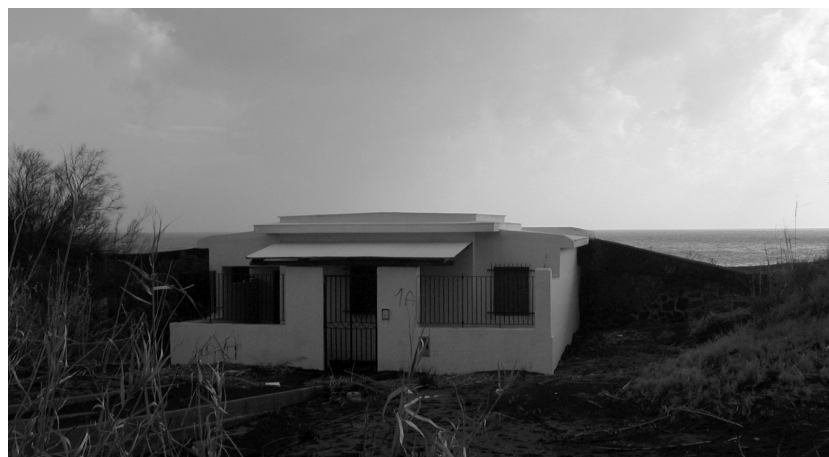
Fig. 13. View of the western side of building #6. The picture was taken a few days after the 2002 tsunami. Building #6 is a Coastguard station on the beach of Scari (Stromboli – Fig. 6). As clearly shown by the picture, the seaward side of the building is totally “covered” by a coastal dune. The PTVA-3 Model attributed to building #6 an “average” RVI score.
