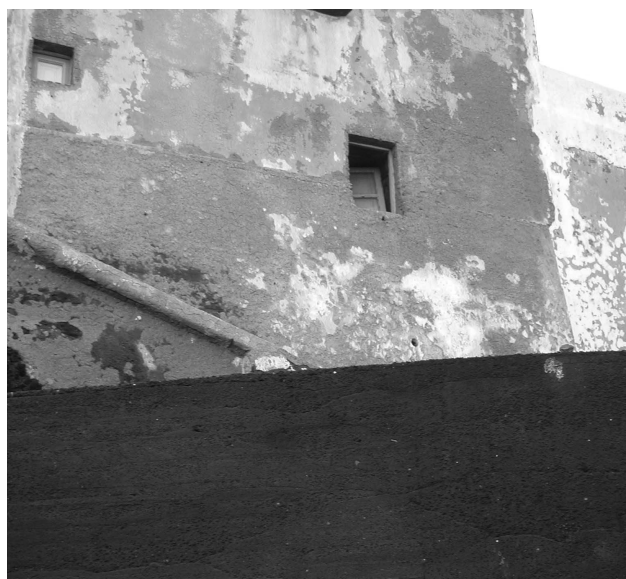
Fig. 8. View from north-west of building #1, at Piscità (Stromboli – Fig. 4). The picture was taken few days after the 2002 tsunami. The only visible damage is an unhinged window on first floor. The PTVA-3 Model classified building #1 as having a “very low” RVI score which correlates well with the actual damage sustained by this building.
