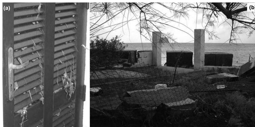
Fig. 11. Two pictures of building #4 (Punta Lena, Stromboli – Fig. 6), taken after the 2002 tsunami. (a) A door on the seaward wall of the building. The inundation did not break it down, but penetrated through the shutter openings and flooded the ground-floor. The building was protected by the vegetation in the front garden (b), some concrete works (a small wall and a table) and by the coastal defences along the shoreline (concrete cubic rocks). The PTVA-3 Model classified this building as having a “low” RVI.
