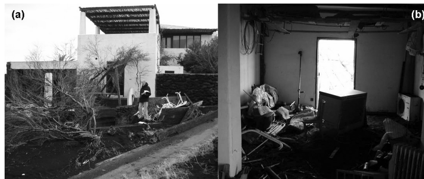
Fig. 9. Pictures of building #2, at the eastern end of Ficogrande (Stromboli – Fig. 5), taken after the 2002 tsunami. (a) A view of the building from north-west. (b) Damage to the interior. The PTVA-3 Model classified building #2 as having an “average” RVI score.
