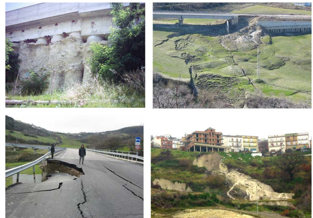
Fig. 2. Damages and failures at Volturino (FG) where housing areas and infrastructures are continuously threatened by landslides.
