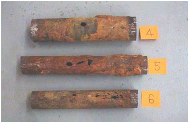
Figure 8. Corroded steel pipes (Greyvenstein and Van Zyl, 2006).
