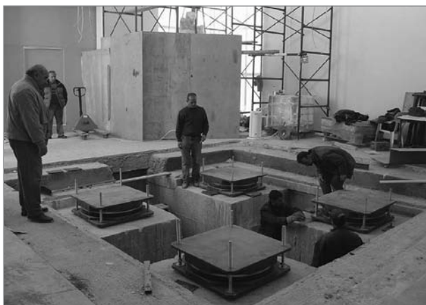
Figure 2: Installation of seismic isolation for the statue of Hermes at the Olympia museum (source: Koumouisis, 2007).
