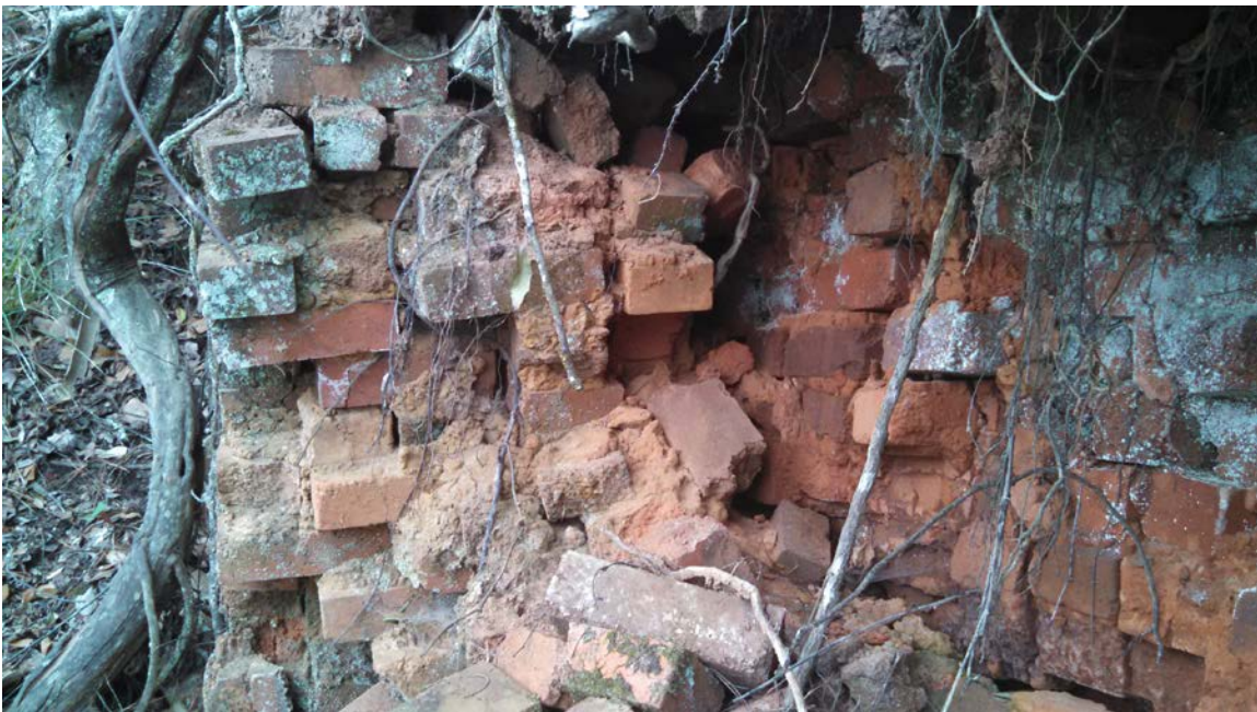
Figure 5.14: Retaining Wall at Landing, Outer Layers of Wall Pulling Away from Bank (Photo Frances Pinto).
