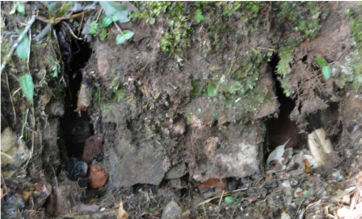
Figure 5.10: Gaps Between Stacks of Bricks (Photo Frances Pinto).
