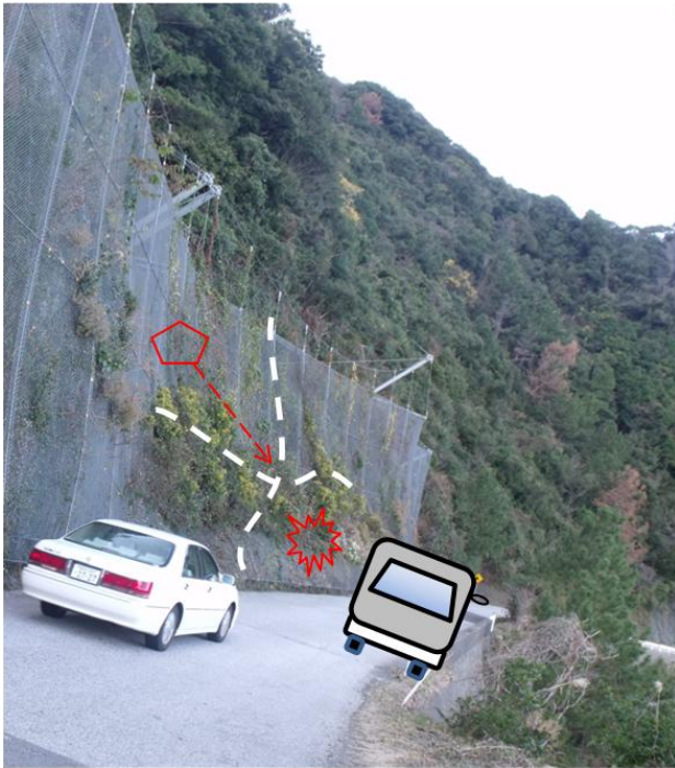
Fig. 4. A simple schematic illustration of the reason for putting the (out-of-plane) displacement response into priority in evaluating the performance of an LPR structure. Actually, the structure is constructed very close to the road-carriageway and the risk onto the road traffic due to a larger displacement of wire-net needs to be checked. Illustrations are drawn over a recent photo of a well-functioning structure from a site along Kurei-Suzaki Line road in Kochi Prefecture of Japan, installed later 2009.
