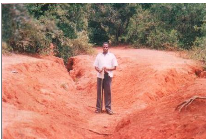
Fig. 4. Gully erosion in Nakasongola district, Uganda
