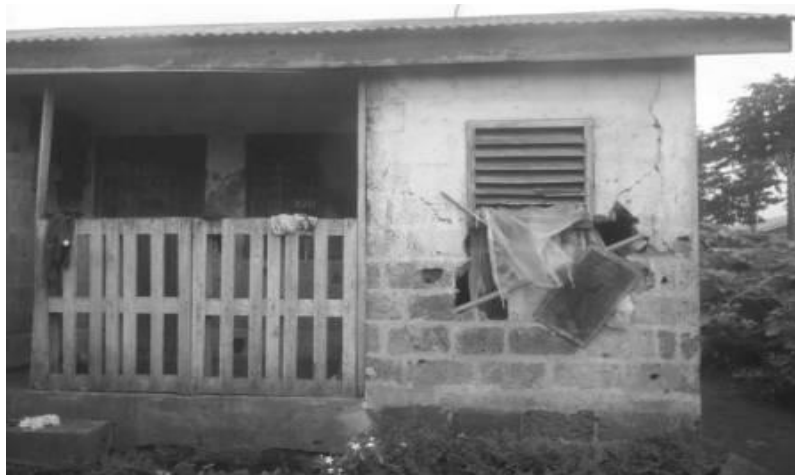
Figure 2. Dilapidated but Occupied Structure in Ekona
