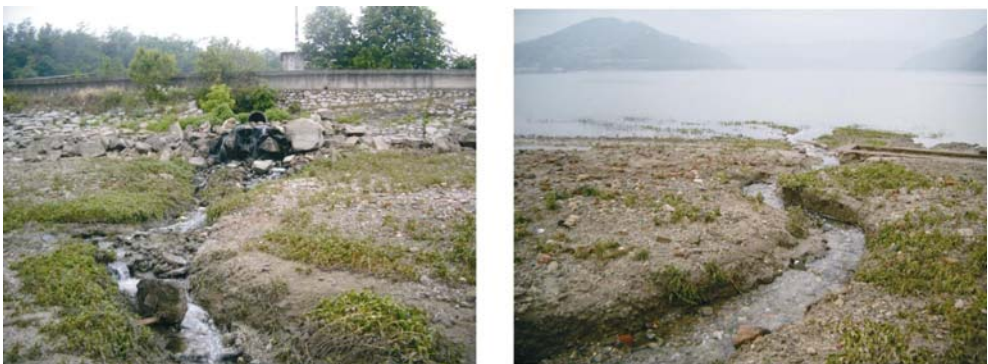
Photo 3. The wastewater discharge pipe at the Sewage Treatment Plant in Orsova town (picture taken in June 2006 when the lowered levels of the reservoir exposed the pipe that normally is submerged). View from the reservoir to the shore (left) and from the shore to the reservoir (right)
