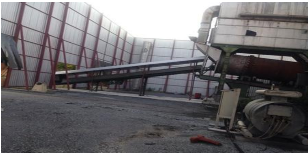
Figure 7: Improvement of Conveyor Belt
