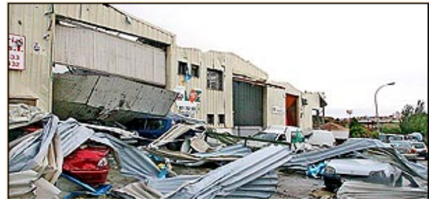
Fig. 2. Damage produced by the tornadoes in the industrial area close to Palma city.
