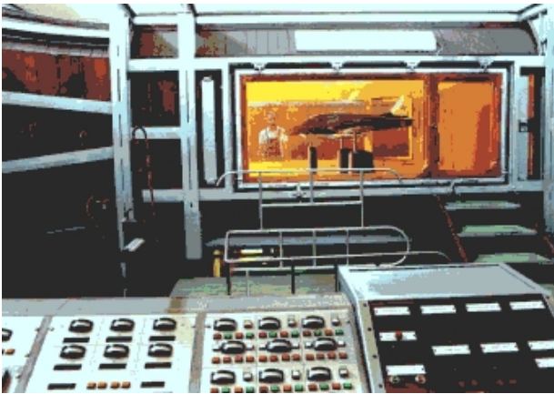
Fig. 2 . The control panel
