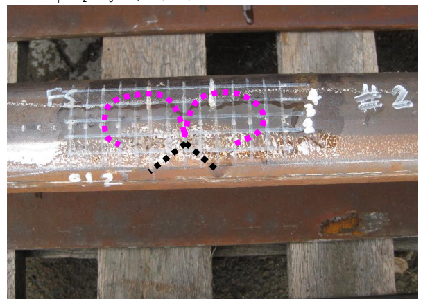
Fig. 10 Ultrasonic testing (Top: crack depths at each grid; Bottom: top view rail surface)
