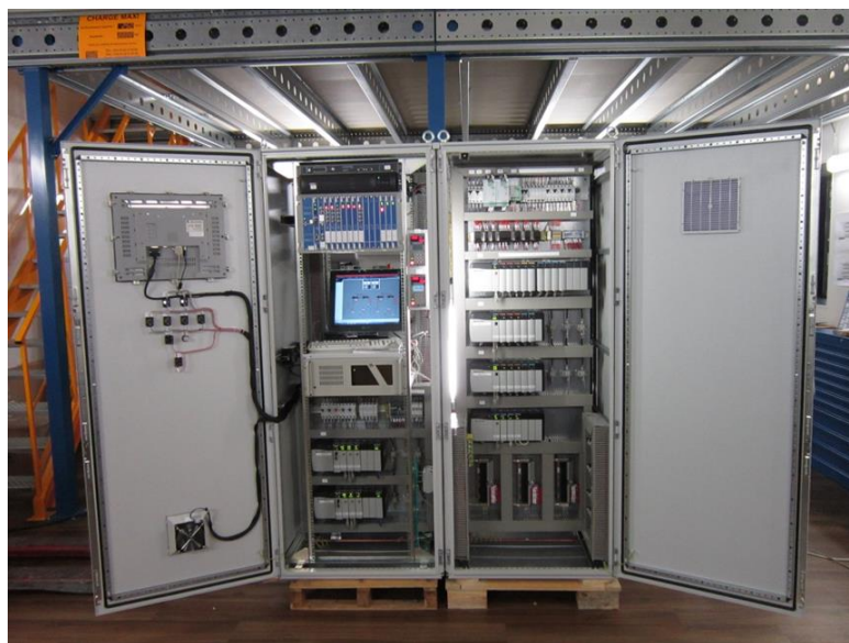
Figure 8 - Typical System Cabinet (Source: Rockwell Automation, Inc.)
