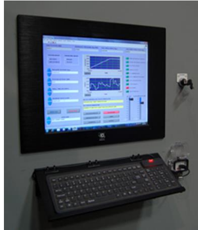
Figure 15 - PLC HMI Workstation
