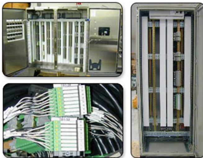
Figure 7 - Typical Marshaling Cabinet
