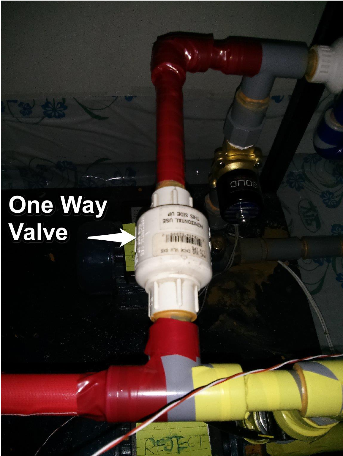
Figure A-5: One Way Valve on the Supply line to Heater
