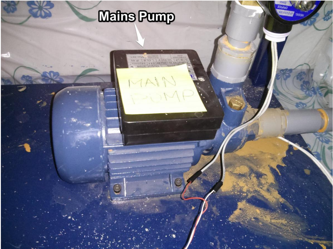
Figure A-3: Water Supply Mains Pump
