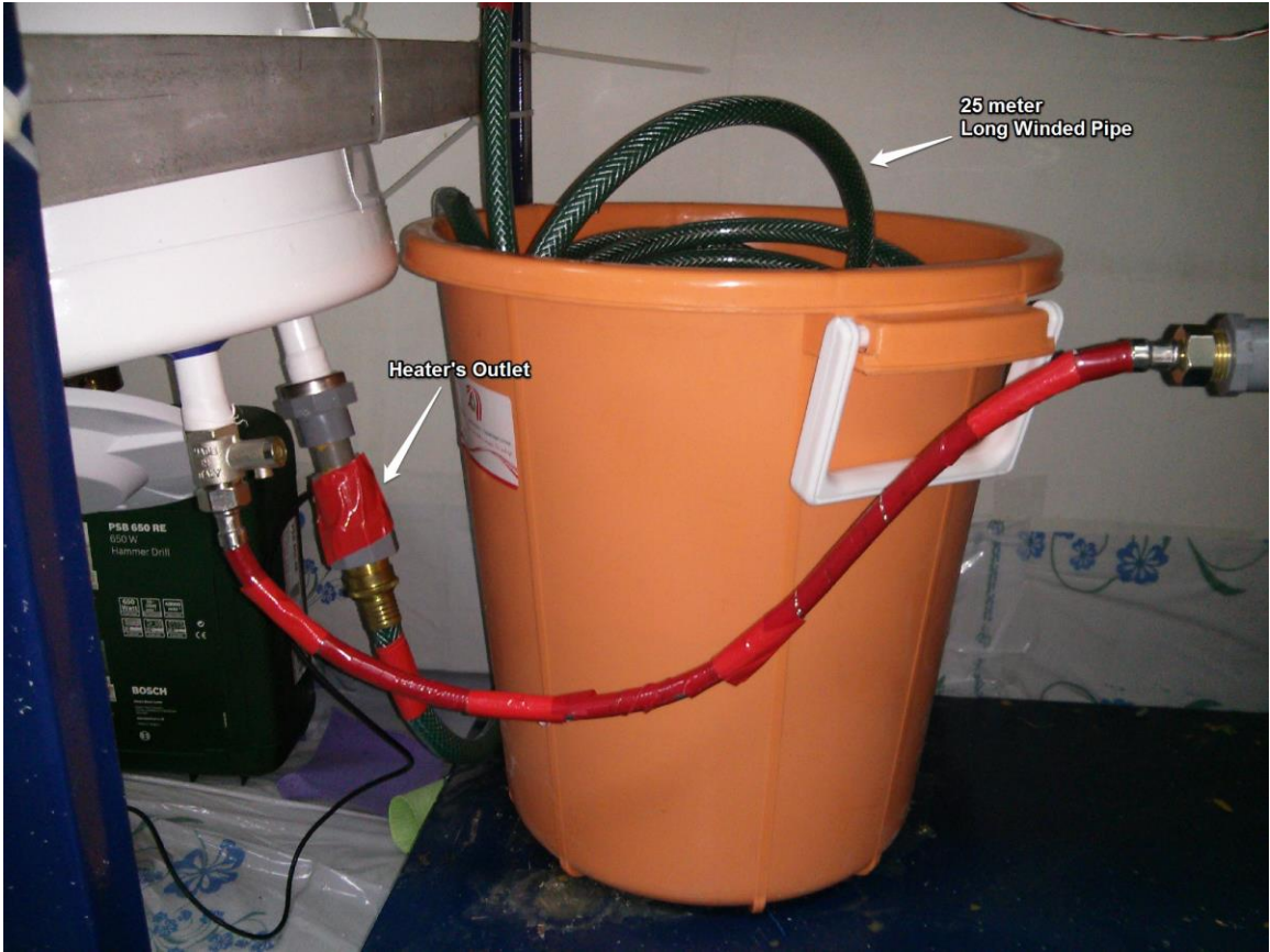
Figure A-10: Heater's Outlet connects to the 25m pipe inside the Orange Container
