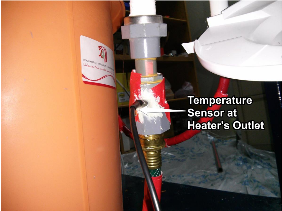
Figure A-8: Temperature Sensor Attached at Heater's Outlet
