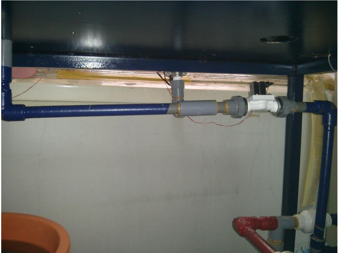
Figure A-17: Solenoid Valve and TEE on the cold line
