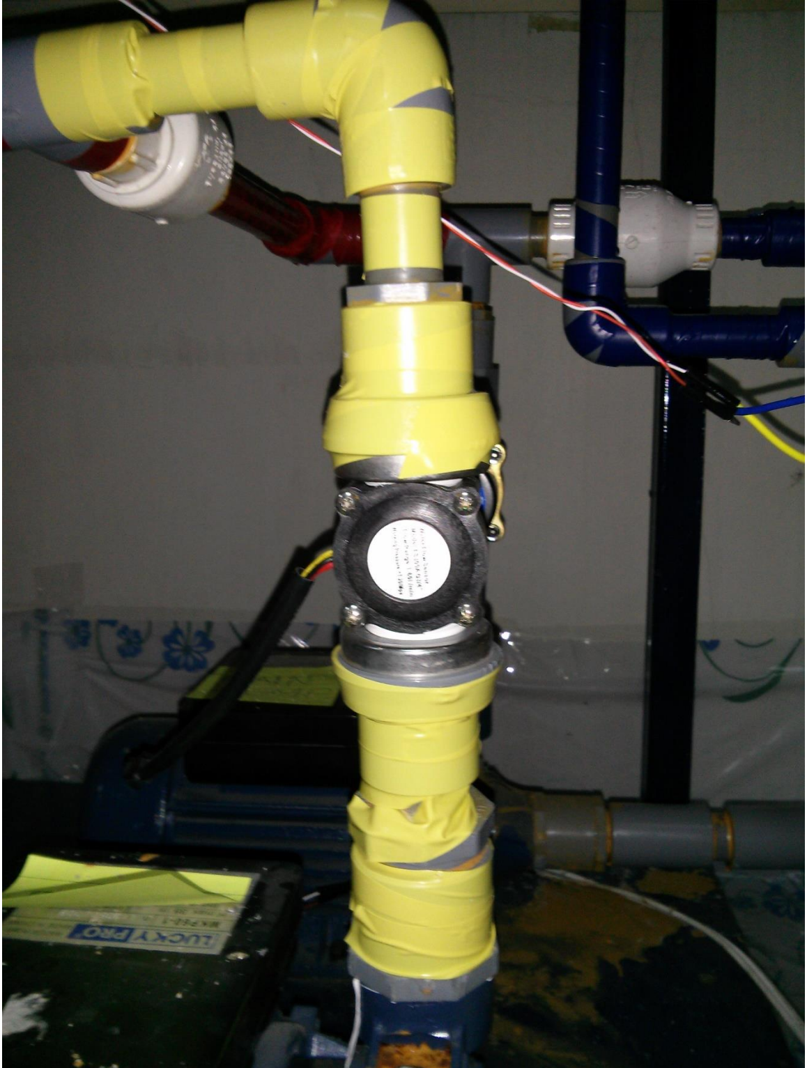
Figure A-15: Flow Meter installed on the outlet of the Reject Pump
