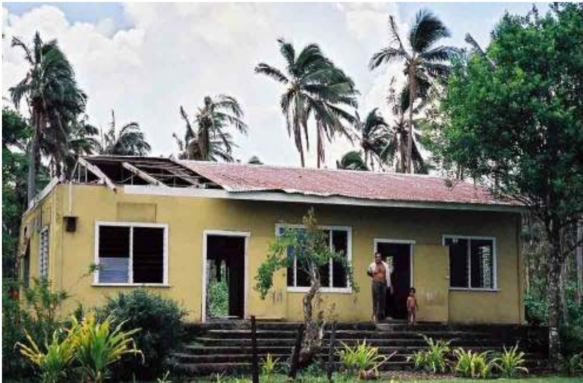
Figure 1: A house on Samoa said to have been damaged by Cyclone Heta in 2004 (photo by Ilan Kelman).
