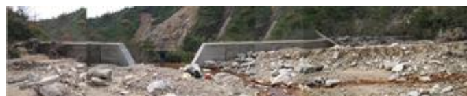
Figure 1. Sediment deposition caused by the closed check dam in the Tsurugi River.
