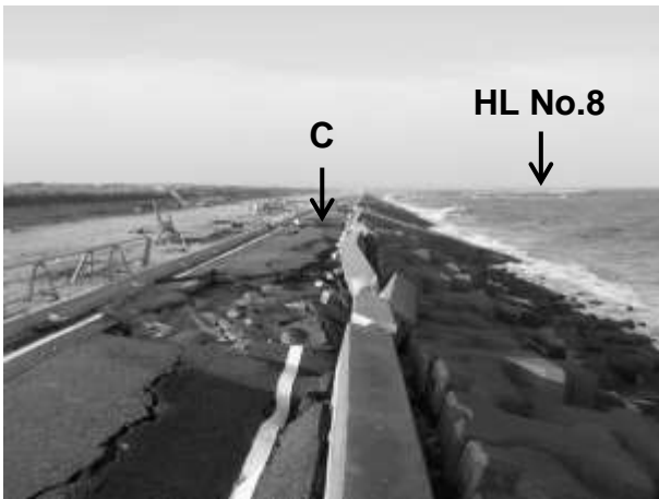
Fig. 9 Damaged seawall on the Node coast.
