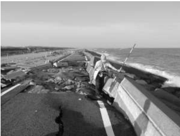
Fig. 10 Enlarged photograph of the damaged seawall.
