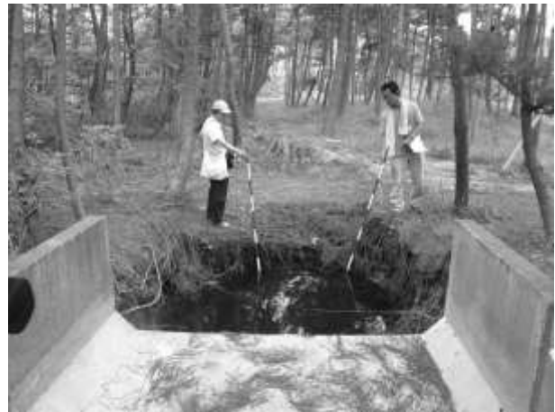
Fig. 21 One meter deep scour hole at the end of a concrete structure.
