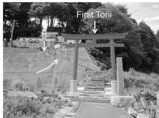
Fig. 4 First torii of Ootsuchi-inari Shrine and many scars left on concrete wall.
