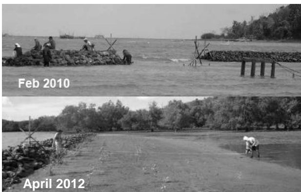
Fig. 14 (top) Breakwaters completed in 2010; (bottom) accreted sediments after 26 months, healthy mangroves seen in the background
