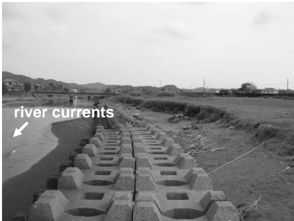
Fig. 6 Subsided concrete blocks and erosion along left bank of Okamoto River (October 13, 2011).
