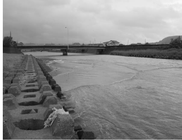
Fig. 8 Concrete blocks on right bank of Okamoto River and sand deposition in front of the concrete blocks (June 11, 2011).
