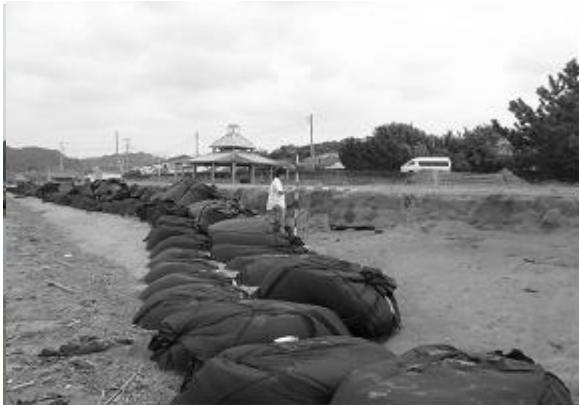
Fig. 11 Severe erosion with formation of scarp immediately north of the river mouth.
