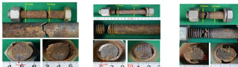
Figure 8: Observation of appearance of high strength bolts
