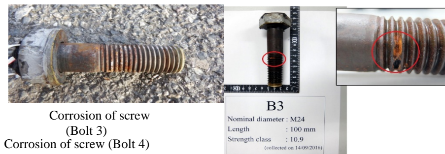
Figure 6: Corrosion of high strength bolts
