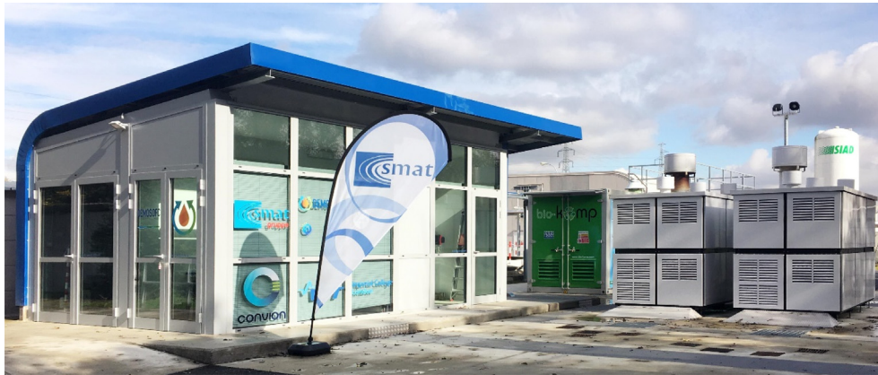
Fig. 12 – DEMOSOFC plant with 2 SOFC modules in operation (December 2018). On the left, the technical building where the control room and the electrical cabinet room are located. In the central part, the first SOFC module. On the right, part of the biogas cleaning and compression container.
