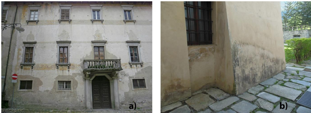
Figure 1. (a) Patches of cement/lime based plaster on historic façade; (b) deterioration (with detachment) of cement plaster applied for the restoration of a masonry subject to moisture.
